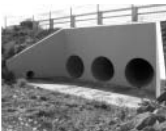
Triple-cell, high bulkhead 1200mm diameter pipe headwall with 450mm diameter pipe in wing wall
