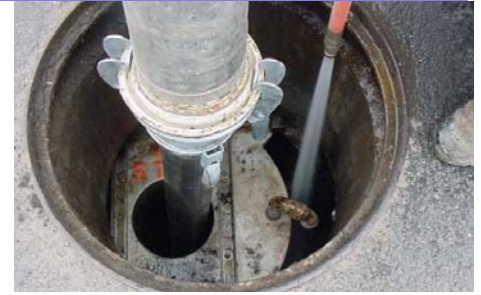
Figure 5 – Vacuuming Sediment Sump
